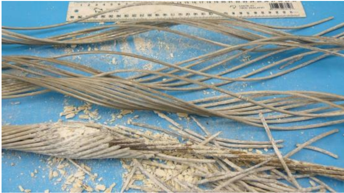
Figure 5: Bulge 1 after removal of the outer layer of aluminium strands, showing the extent of internal damage of aluminium wires
