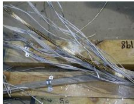
Core exposed and no grease (white patches)
