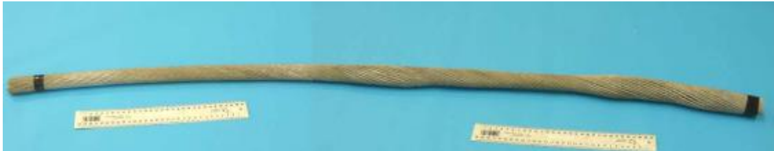
Figure 3: Sample of conductor showing two bulges that are relatively large, but extremely difficult to see in span from ground.
